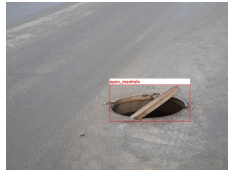
OPEN MANHOLE Fall risk on public right of way
